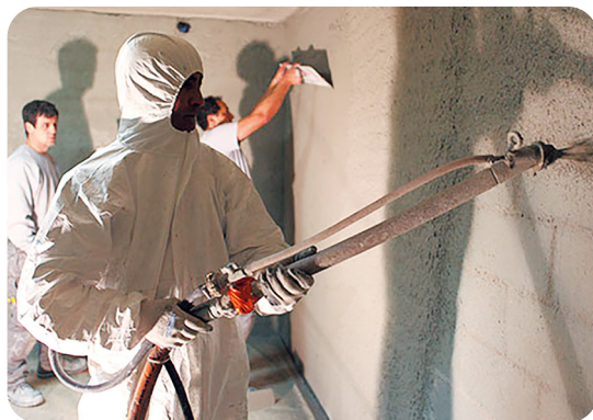
© Hydrotec assainissement Wavre
